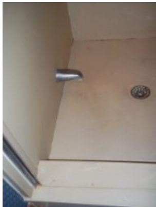
Faucet too low.
