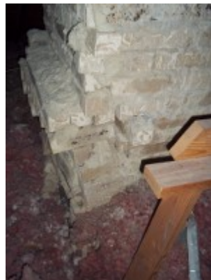
Chimney has gaps in attic.
