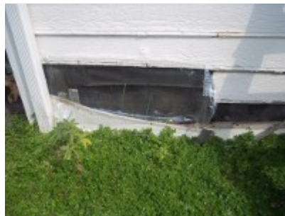
Missing wall boards.
