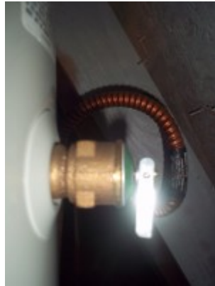
TPR valve line going up.
