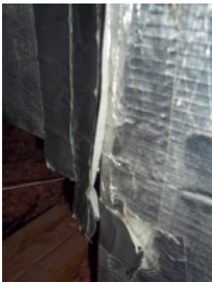
Plenum improperly sealed.
