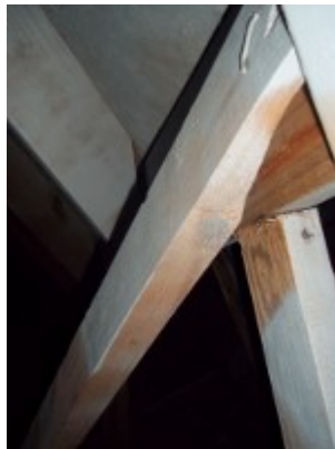
Brace not attached.
