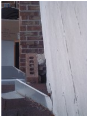
Columns open at top allow water entry.
