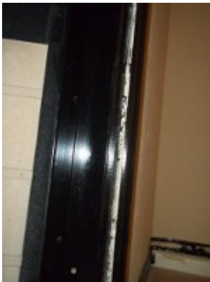
Gap by fireplace to the wall.
