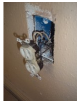
Outlet not attached.
