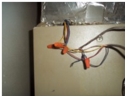
Wiring connection not in unit.
