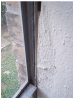
Moisture damage to wall in window area.
