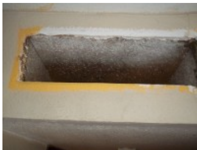
Missing vent cover.
