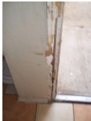
Missing trim front door.
