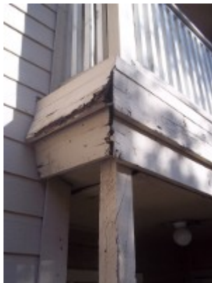
.Moisture damage porch area.
