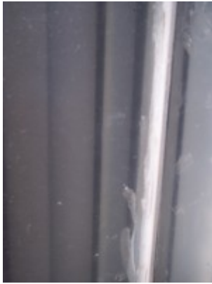
Window glazing strip missing.
